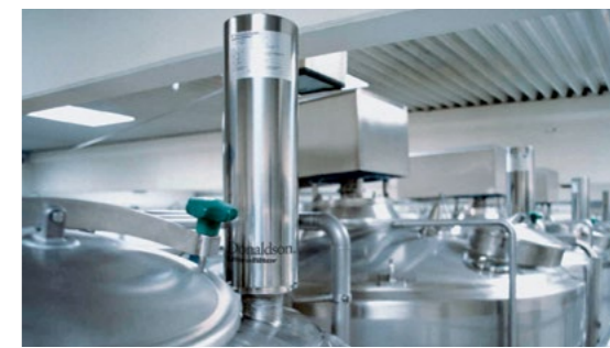
Filter housings for the aeration on storage tanks
